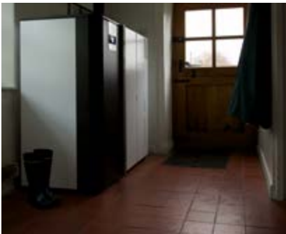
44 UTILITY WOOD PELLET BOILERS
